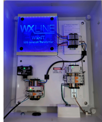
Wxline Isolation Transformer (WxIT) in Fiberglass Enclosure
