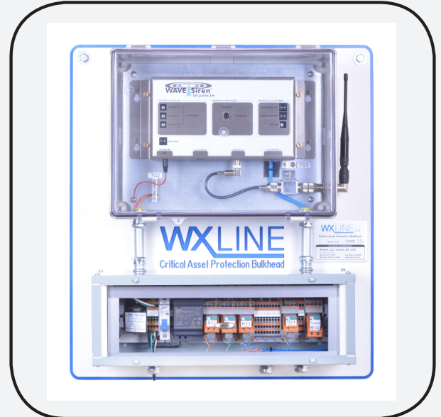
CAPB-PUMP with WAVE Sequencer and switch-gear.
